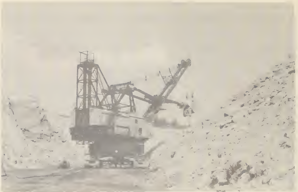
Figure 5.--Strip-mining by power shovel methods accounts for more than 50 percent of the area stripped for coal in the Central States.
